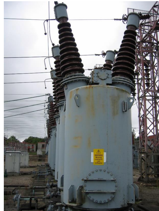
Catterson, Victoria. 132kV Circuit Breaker. [Photograph]. Retrieved from https://www.flickr.com/photos/cowlet/36524280/
